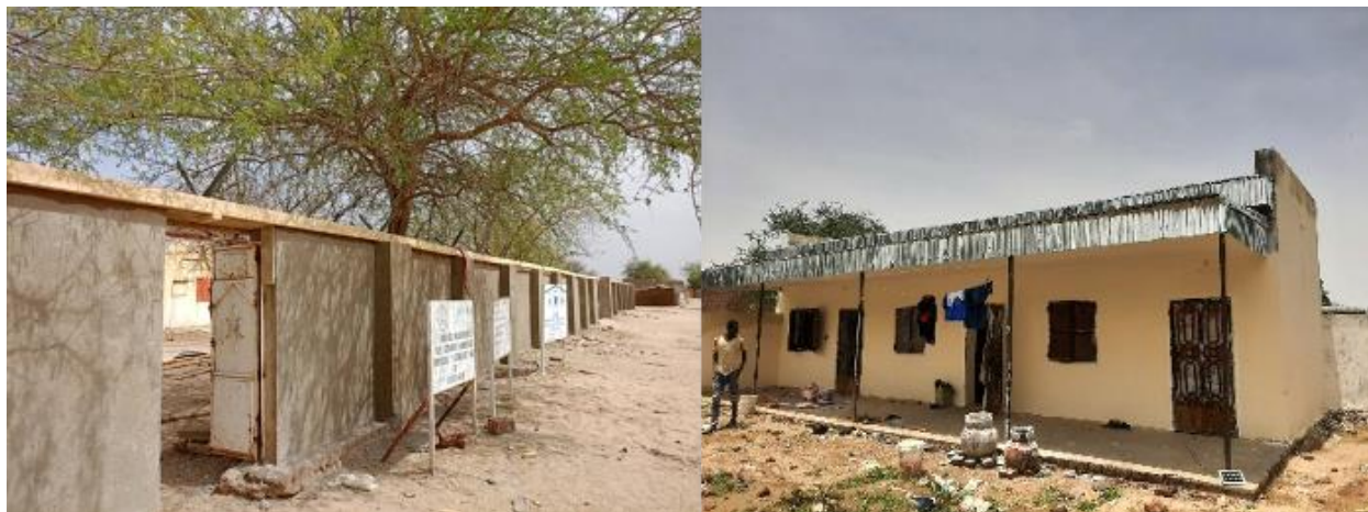
Figure 4: The barrier and base camp being restored at the Hadjer Hadid Branch, Chad
