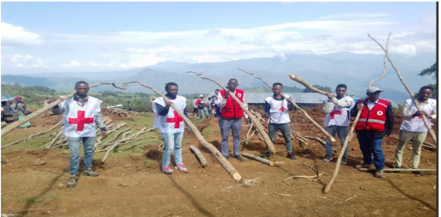
ERCS volunteers mobilized other local volunteers to support emergency shelter construction to relocate people affected by landslide in Gofa. Photo credit, ERCS zonal branch.
