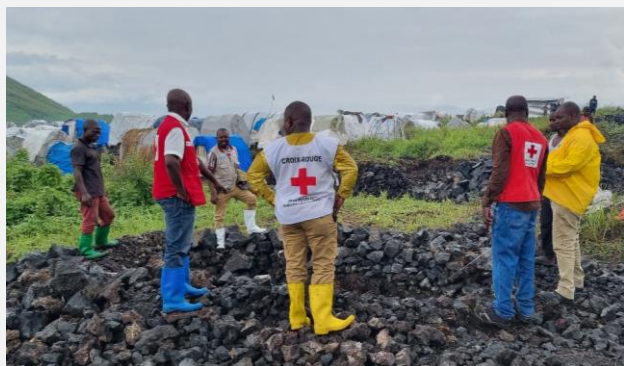
The logistics and WASH team from the North Kivu branch, supervising the latrines under construction in Lushagala.
