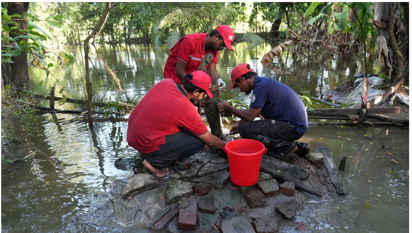
BDRCS volunteers were repairing a water point in a flood-affected area of Noakhali district. (Photo: BDRCS)
