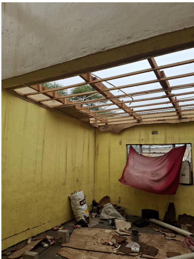
Picture shows extent of damage to residential property in Kgaphamadi
