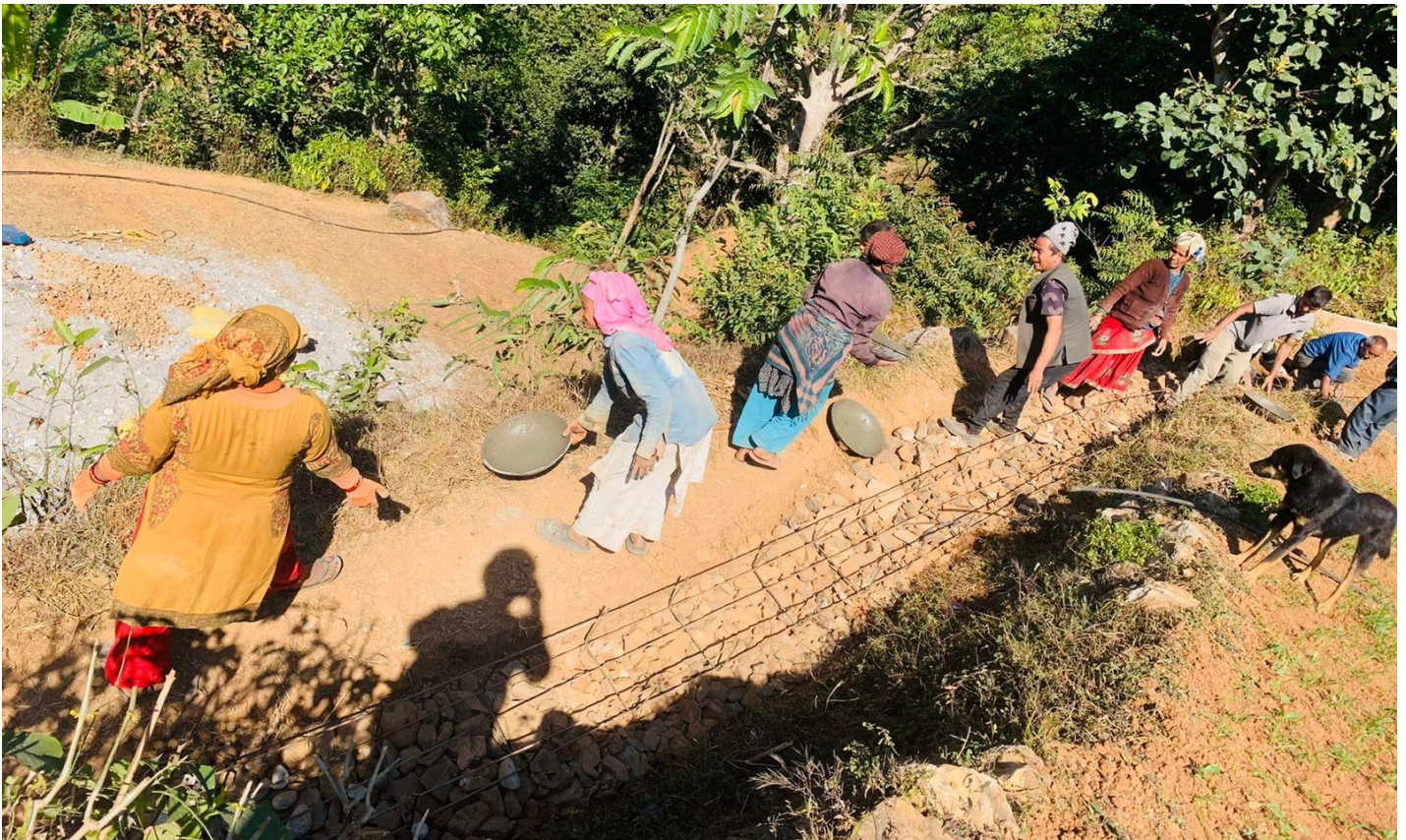
Community people participating in the cash for work activity as part of the livelihood support to construct an irrigation canal in Salayn District (Photo: NRCS)
