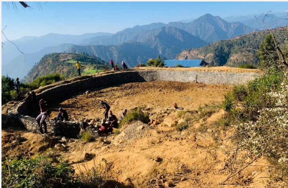
Water recharge pond being constructed in Rukum West District as part of the mitigation activities. (Photos: NRCS)
