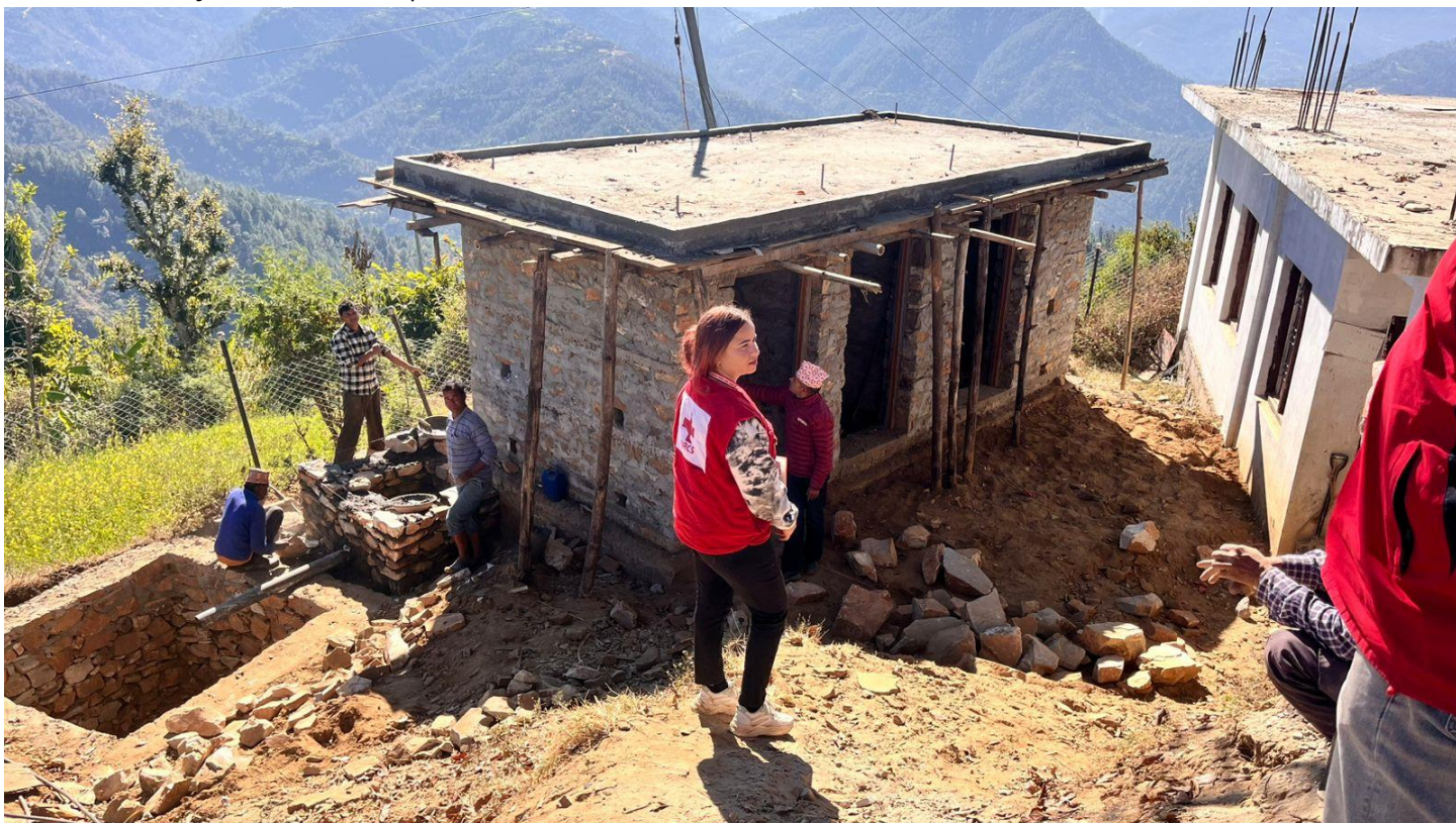
NRCS staff monitoring the toilet construction process in one of the targeted districts. (Photos: NRCS)
