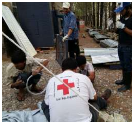
The Spanish Red Cross sanitation ERU working with local community members and NRCS volunteers to construct emergency toilets. (Photo: NRCS)
